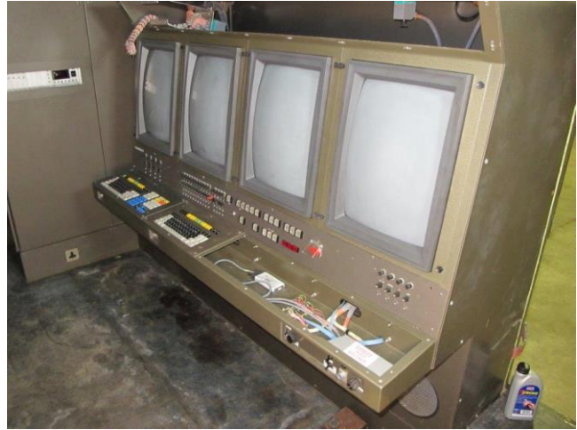
Display Console with missing top switch panel and Engagement Controller's keyboard
